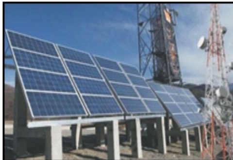
SOLAR POWERED TELECOM TOWER
