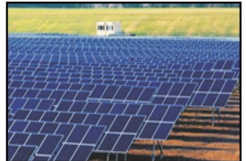
UTILITY SCALE SOLAR FARMING
